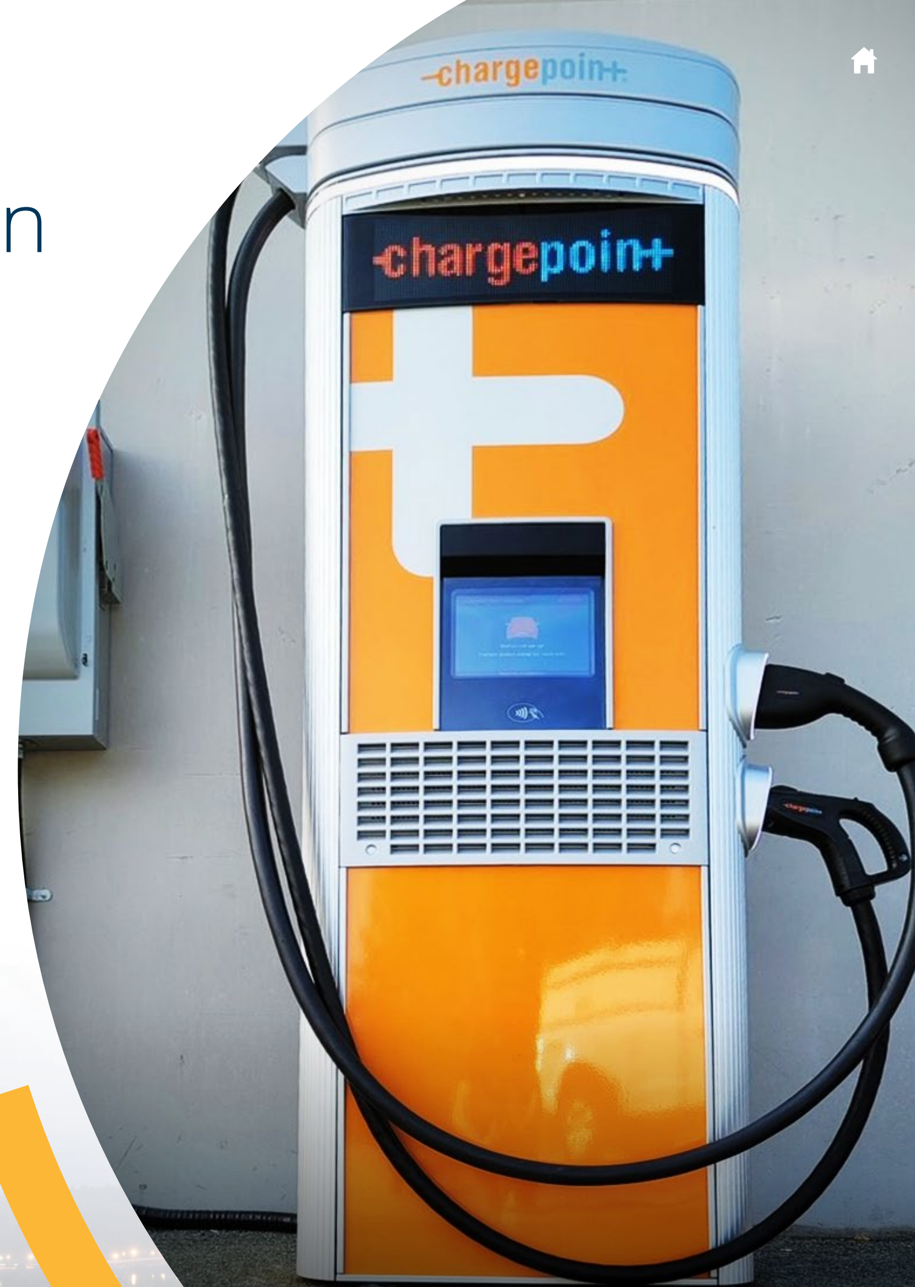
Photo Source: QuadReal, EV Charging Station, Park Place, Vancouver, Canada
